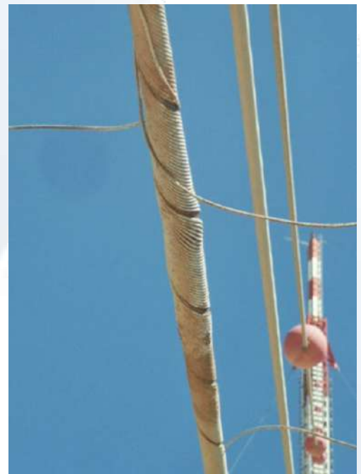
Broken guy wire strands
