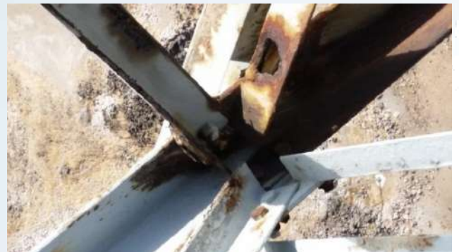
Heavy rust on coastal structures
