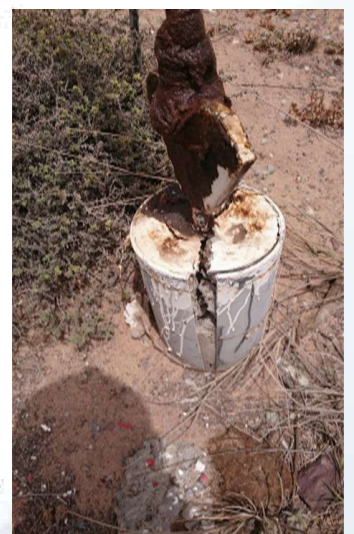
Cracked concrete due to rust expansion on anchor plate
