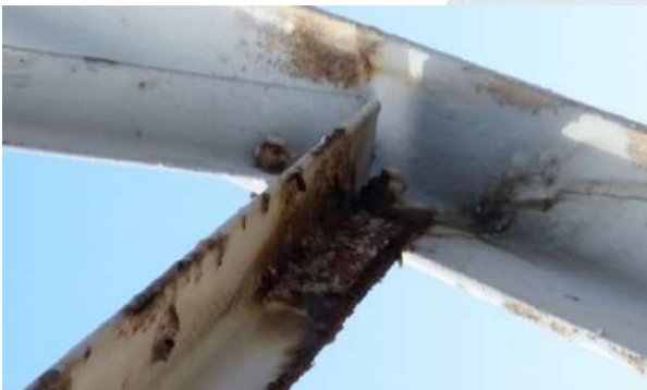
Heavy rust on coastal structures
