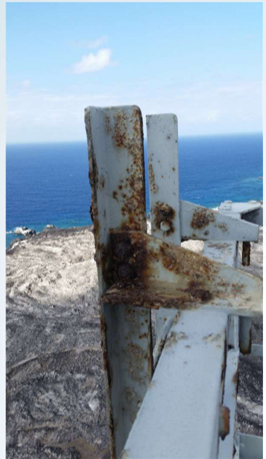
Heavy rust on coastal structures
