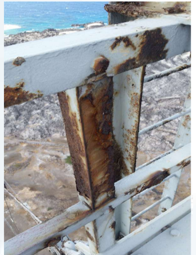
Heavy rust on access platform
